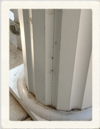
A Column Before Cleaning
